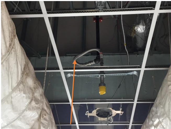
Failing to maintain the 4" minimum radius & number of bends allowed for 2' hose in violation of the U. L. Listing.
